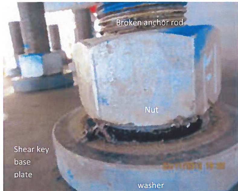
(a) One of failed anchor rods on a shear key base plate
