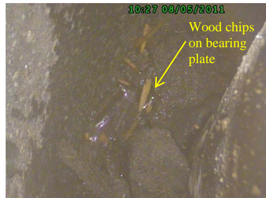
Figure 10: Various Debris on the Bearing Plate
