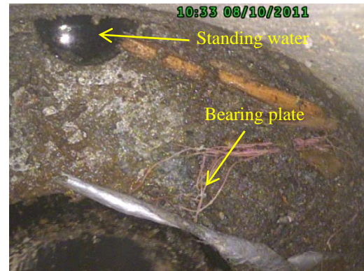
Figure 12: Various Debris on the Bearing Plate
