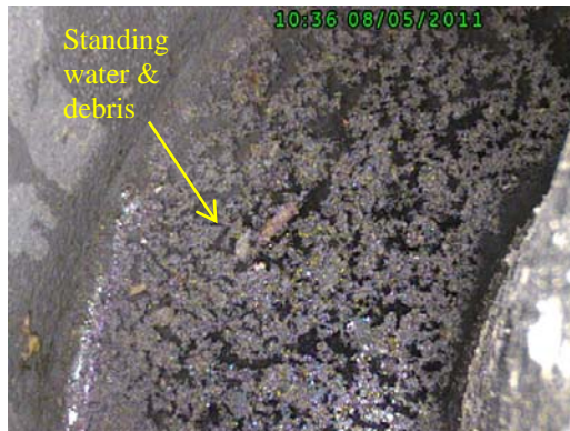
Figure 11: Standing Water in the Rod Hole
