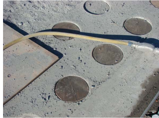
Figure 6: Capped Rod Holes
