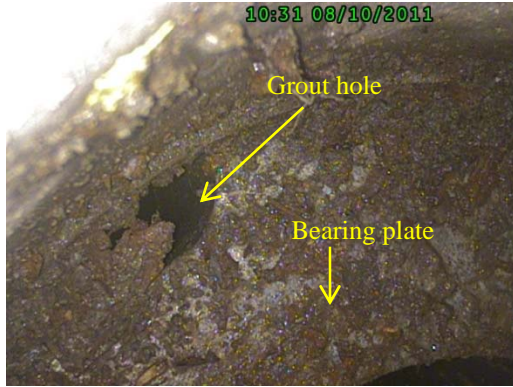
Figure 7: Grout Hole Blocked
