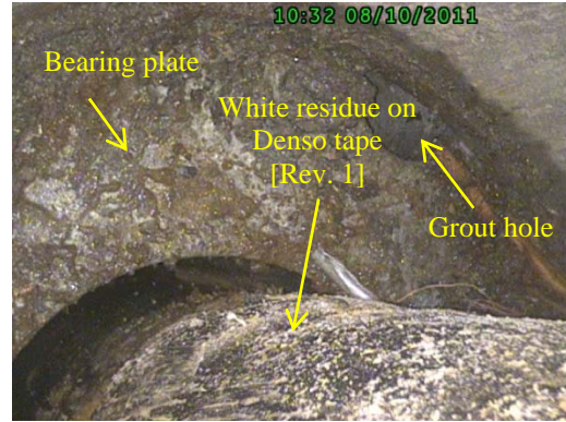
Figure 8: Debris on the Bearing Plate
