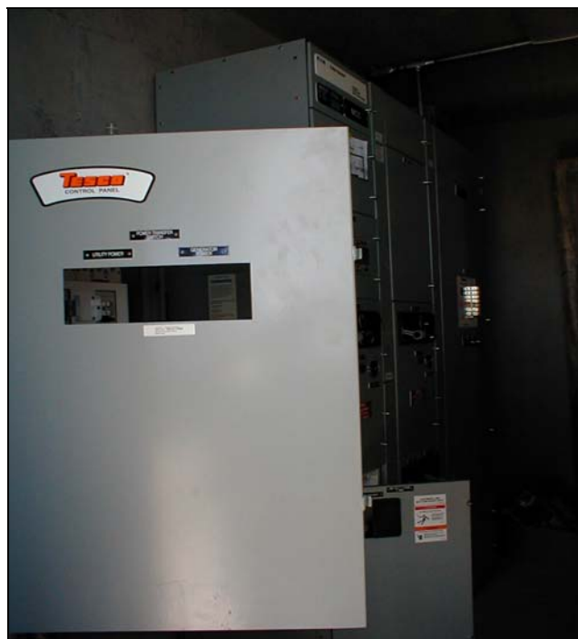
Area 5, Substation 6, - Tesco Control Systems
