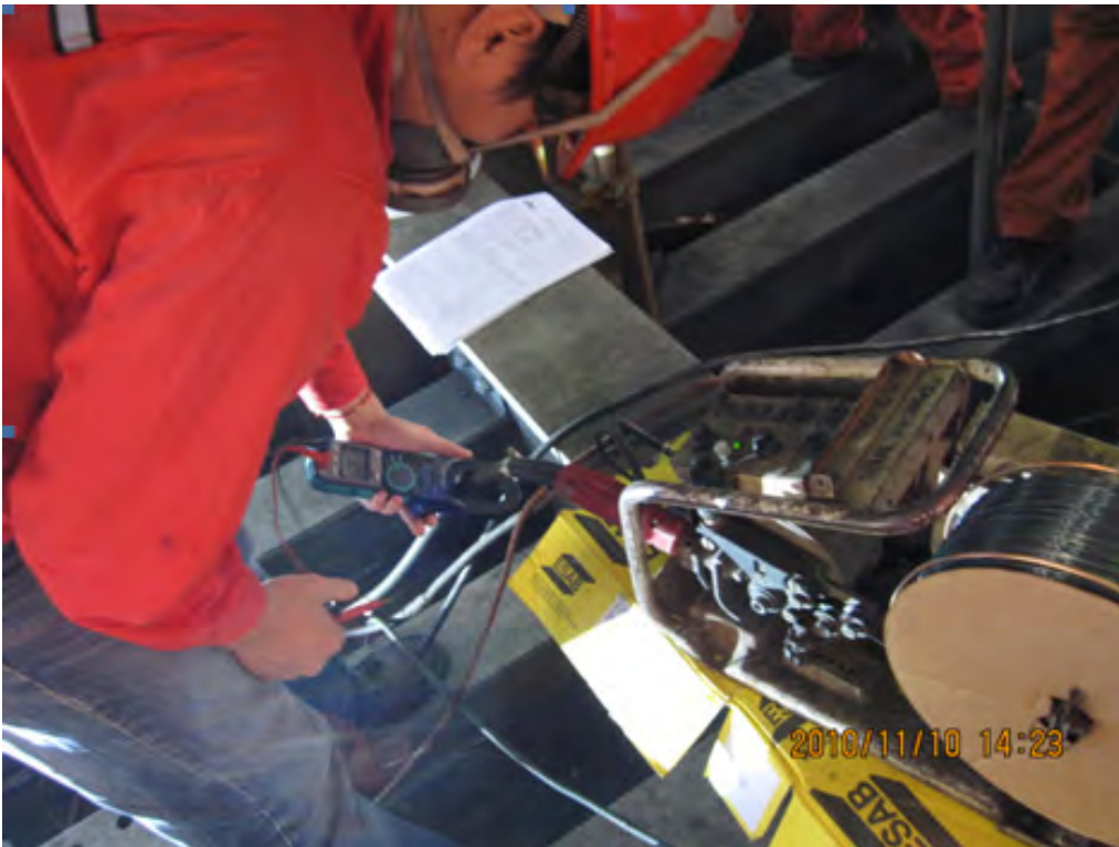
SAS ESAB Wire Being Used for the First Time on Lift 11 Welds
