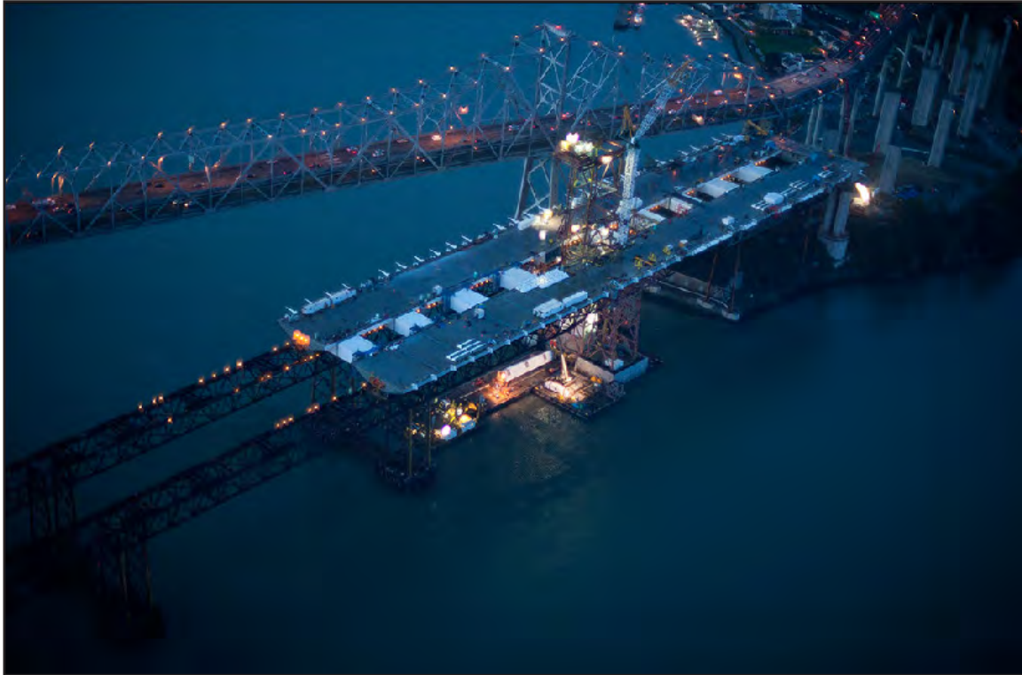
SAS Aerial View of the Shear-Leg Crane Barge Erecting the Tower Lifts
