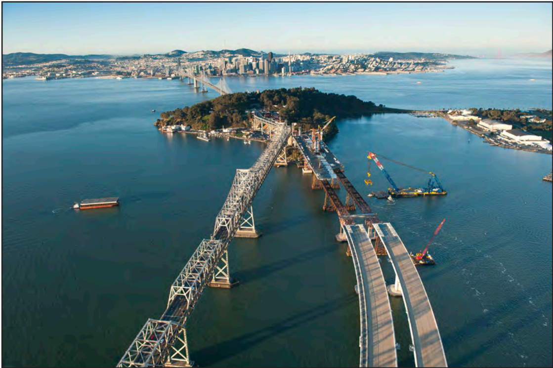
Shear-Leg Crane Barge (on right of bridge) Awaiting Arrival for a Roadway Box (being pulled by tugboat on left)
