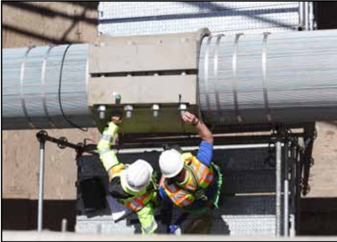
Verifying the initial Length of the Cable Band Bolts on the West Loop of the Self-Anchored Suspension Bridge
