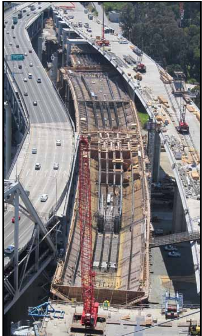
Yerba Buena Island Transition Structure #1 Westbound Deck Complete and Eastbound in Progress with Existing Bridge on Left
