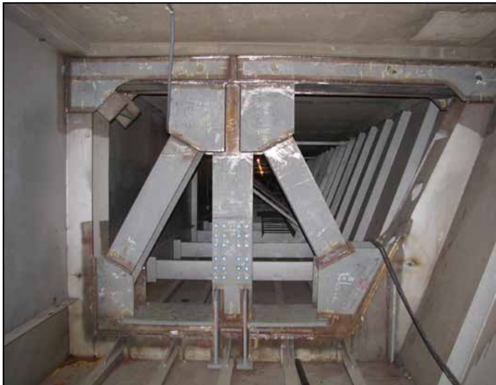
Pier 28 Jacking Frame
