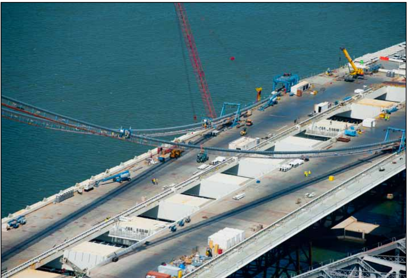
The East end of the Cable Compaction Shows the Remaining Area to be Compacted
