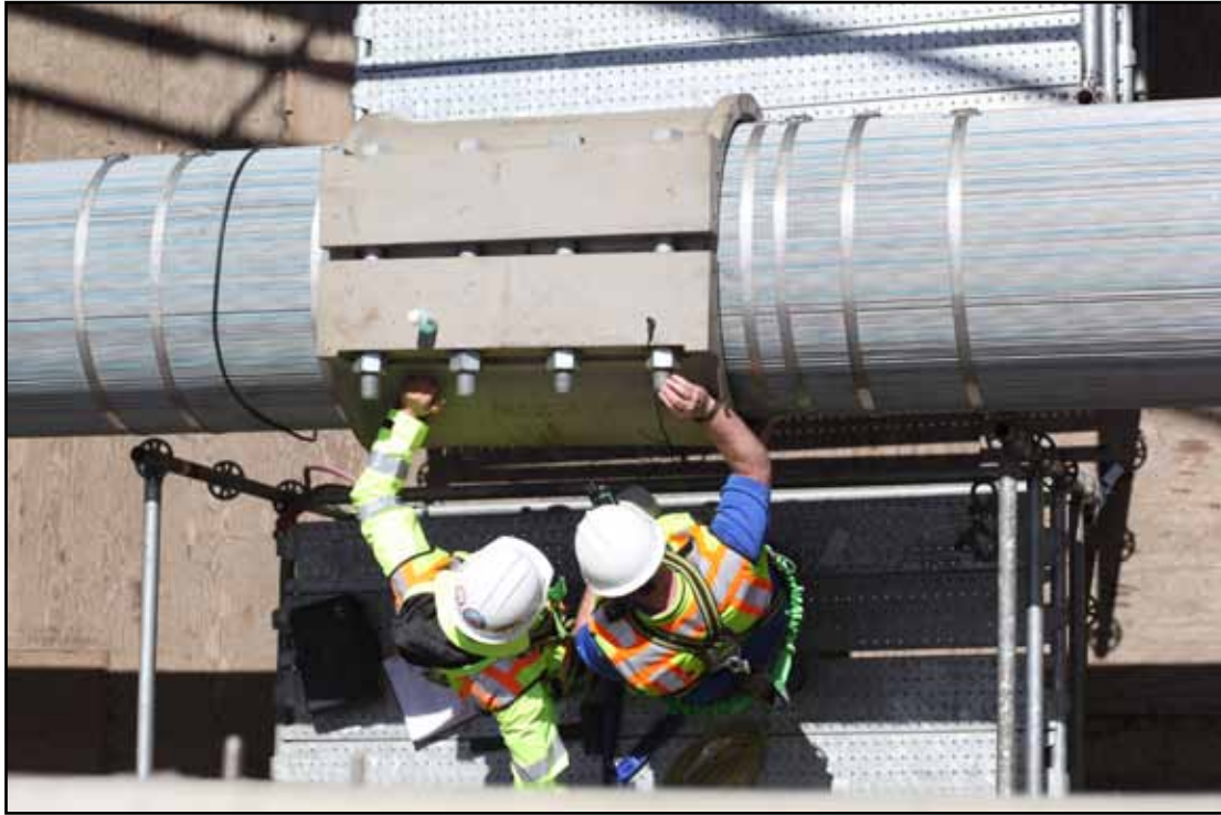
Verifying the Initial Length of the Cable Band Bolts on the West Loop
