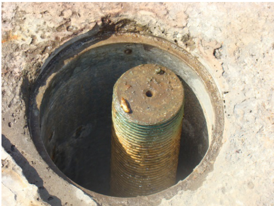
Figure 2.1-6: Exposed Rod at Pier E2
